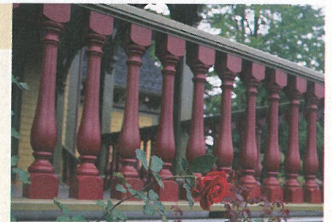
Millwork companies can easily recreate antique woodwork. These balusters and railings were modeled after those found on the porch of a 19th-century home in Rhode Island.
